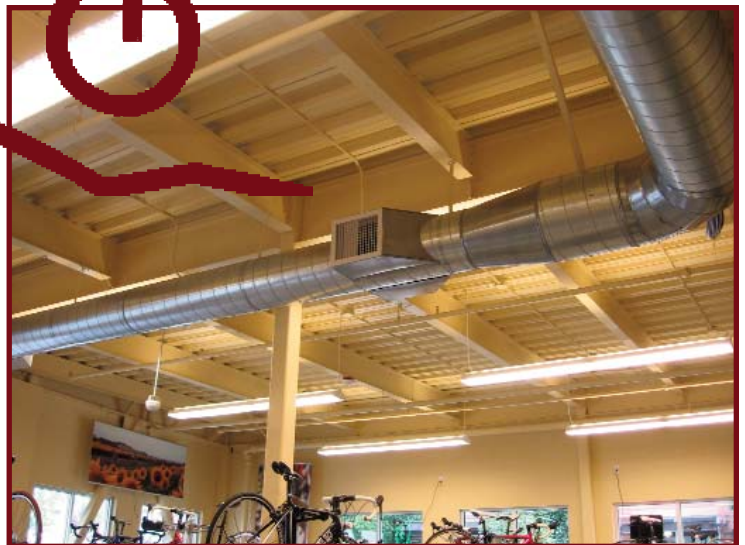
Exposed metal roof decks have replaced standard drop ceilings, which would potentially help in reducing the echo in the space.
